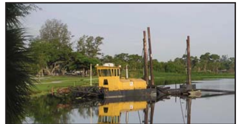
The 10-inch dredge used by American Earth Movers to feed the dewatering system at about 2500 gallons per minute of a slurry containing 15 percent solids.
